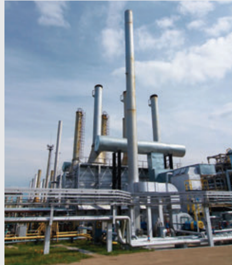
Natural gas processing facility.
