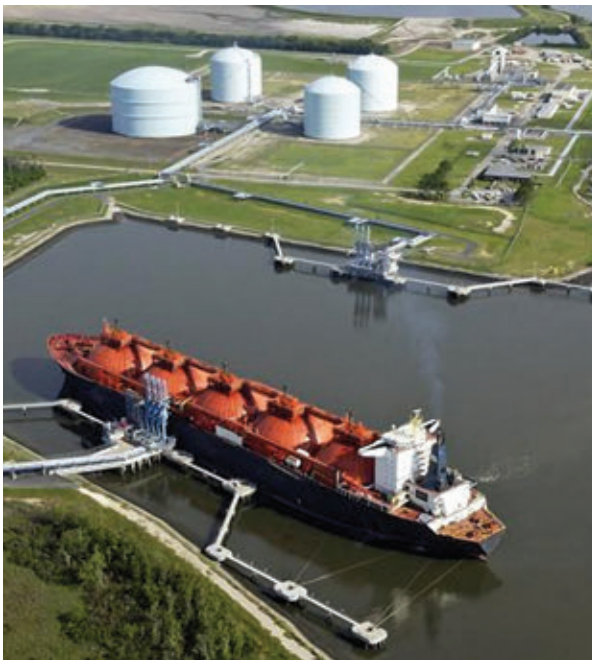
Insulated Low Pressure Storage Tanks for LNG
