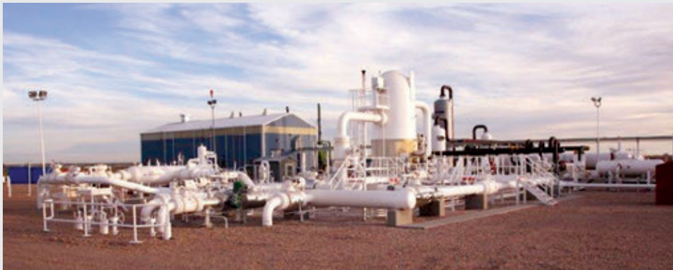
Natural gas compressor station.
