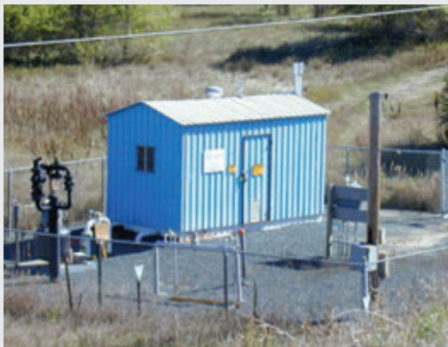
City gate meter station.
