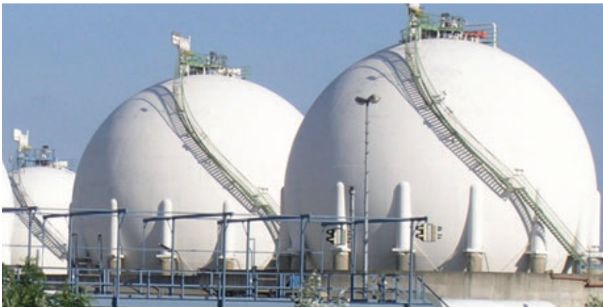
Compressed Natural Gas
