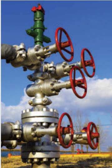
Natural gas wellhead.
